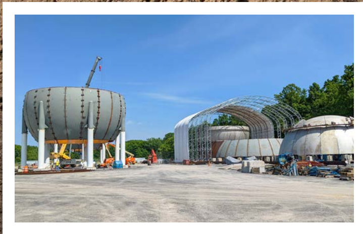
Caption: On October 20, 2021, Governor Hochul announced leading alternative energy technology provider Plug Power has begun construction on a $290 million electricity substation and green hydrogen fuel production facility at the WNY STAMP site in the Town of Alabama, Genesee County. (Photo Credit: Mike Groll, Office of Governor Kathy Hochul)
